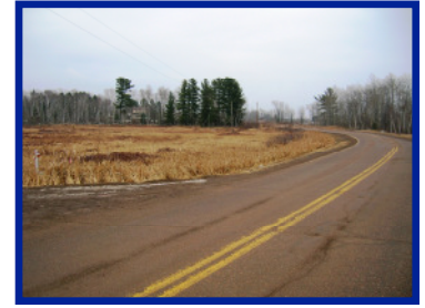
A portion of the county road needing reconstruction.
