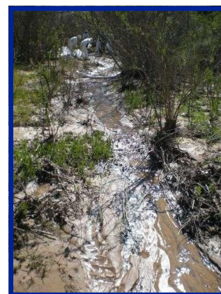
Two workers trying to contain Greka oil spill in creek Photo: SBFDF
